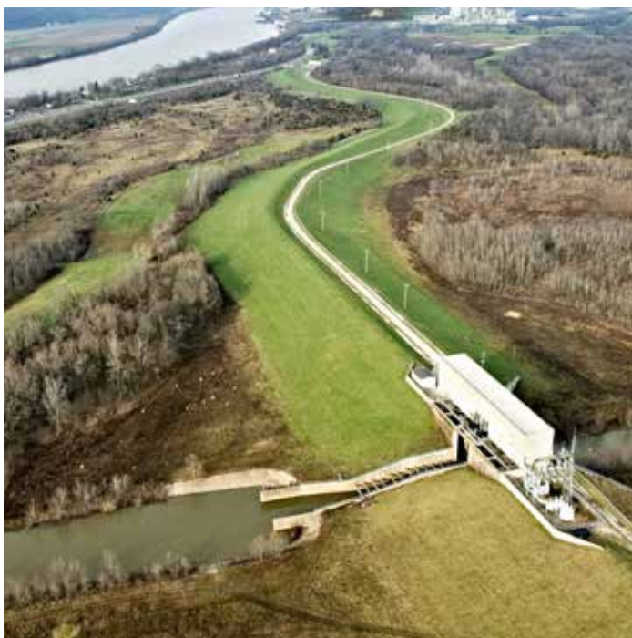
Two Pumps at the Pond Creek Flood Pumping Station that were damaged during the February/March 2018 flood are to receive repairs in the next 12 months.
