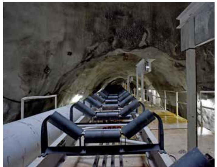
This conveyor system allows removal of the excavated rock as Bumblebee's cutterhead buzzes through 4 miles of rock.
